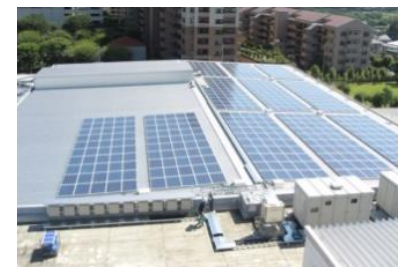
Solar power generation system
