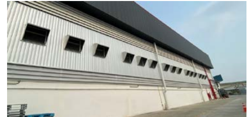
Newly installed ventilation ducts in Janome Thailand Co., Ltd.
