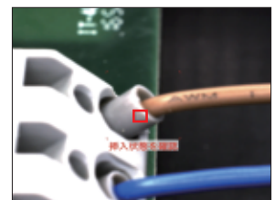
Cable Insertion Status
